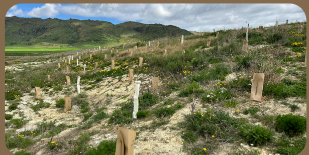
West Race Slip remedial work & planting of poplar poles and natives for bank stabilisation
